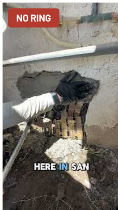
"A" for effort on the stucco patch
