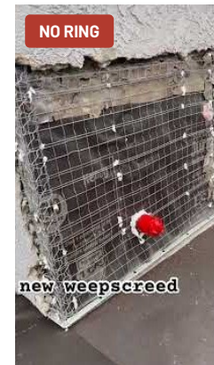
Stucco repair due to broken water pipe
