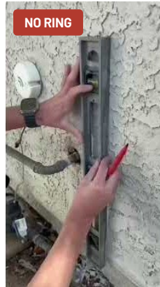
Found a Pinhole Leak in Main Water Line! Cutting Through Stucco Wall
