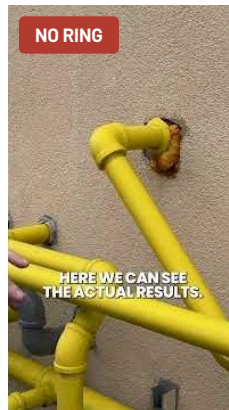
Small holes around pipes can turn into big stucco problems
